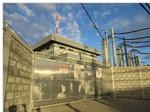
Balagtas 115 kilovolts (kV)-34.5 kV Substation
